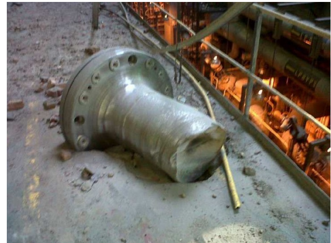
Eskom (Sth Africa) Duvha Unit 4, Feb. 2011 Overspeed test failure
